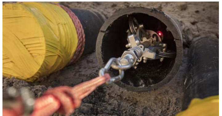
DuctRunner in leiding
